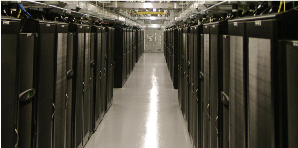
Courtesy: Massachusetts Green High Performance Computing Center ( mghpcc.org )
